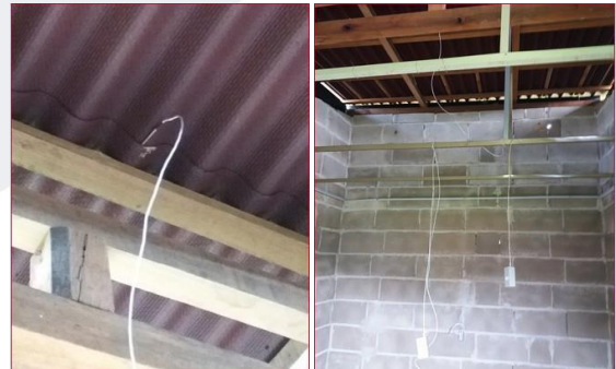
Thermocouples installed in building with Onduline roof
