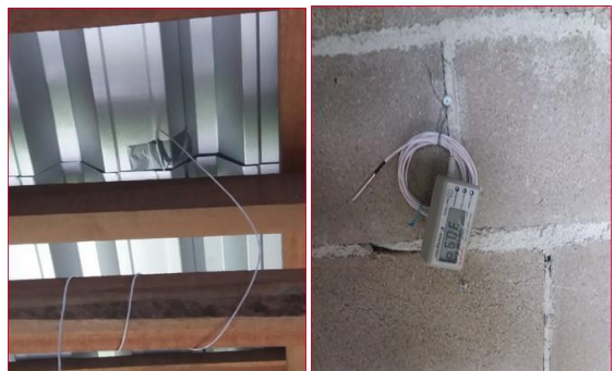
Thermocouples installed in building with metal roof
