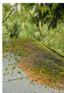
FIG 4 - Moss growing on leaf debris on shaded felted roof. Moss thrives in shaded damp conditions
